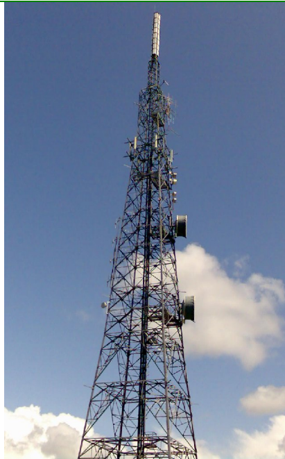
Transmitter Site Photo
